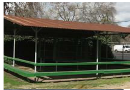
REPAIRS—The roof of the Bingo Stand needs a power washing and fresh paint—SPA will buy the paint—need equipment & People Power!
